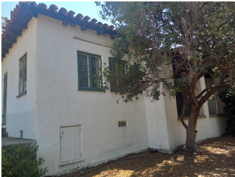
Photograph #21 Property at 3935 Thacher Road North end of west elevation (Looking SE)
