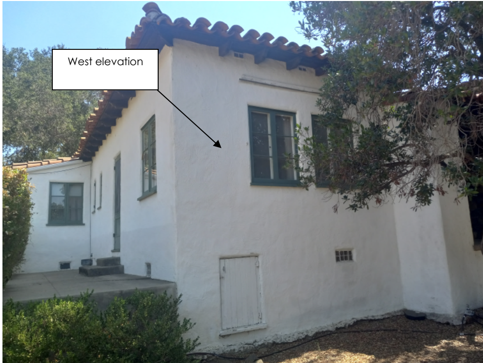
Photograph #20 Property at 3935 Thacher Road North end of west elevation (Looking SE)
