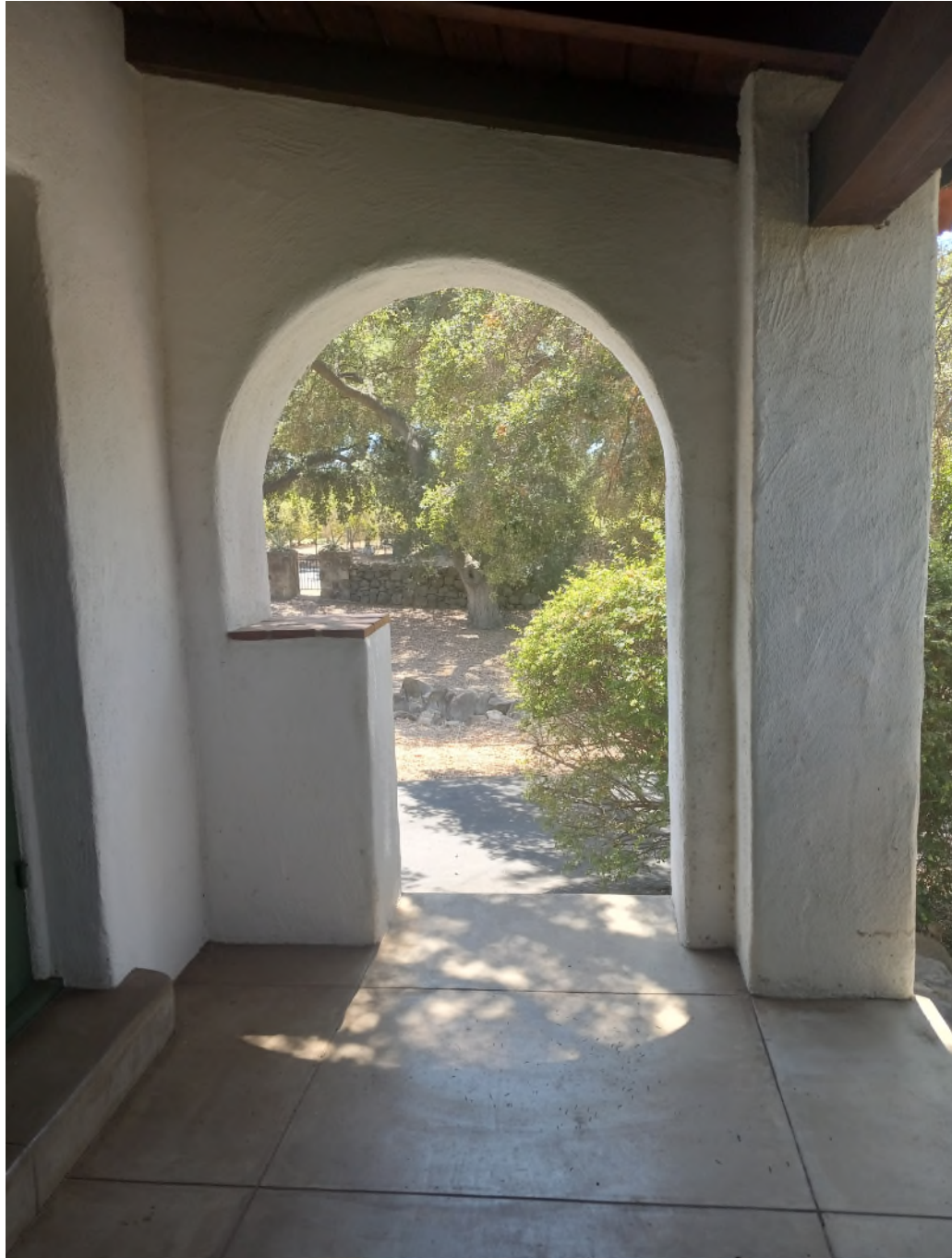
Photograph #24 Property at 3935 Thacher Road Detail of the front porch on the west elevation (Looking south)
